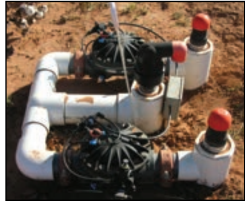
Figure 3. Example of a field installation of pressure regulating valves and air vents
